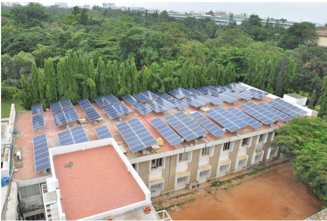
Figure 4.2: Solar panel structure on the main building at Bengaluru
